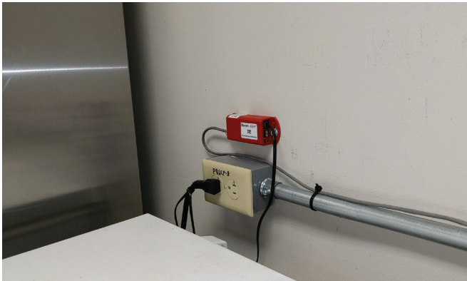
Room Alert 3E used by LifePath
